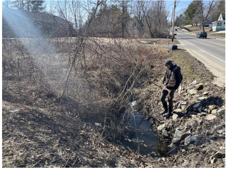
Photo 10. View north of Ditch 1 where it enters the culvert under South Main Street.
